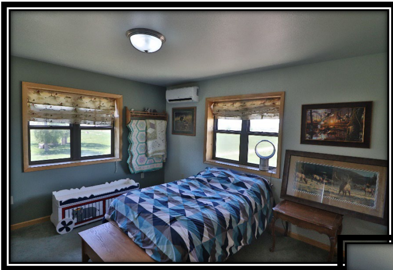
Guest Suite On Main Level Heat pump for heat and AC
